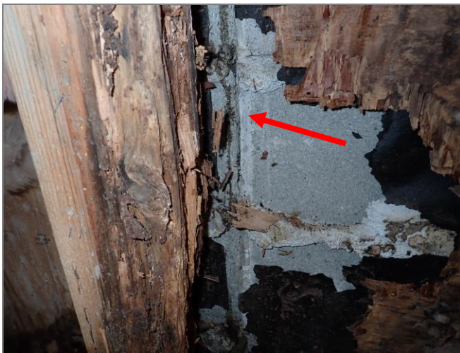
Water was also observed entering through an open joint in the CMU block veneer.
