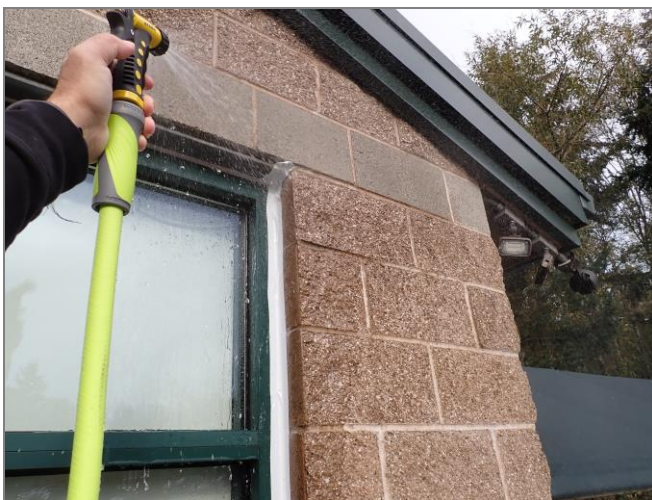
Water applied at the head of the window.
