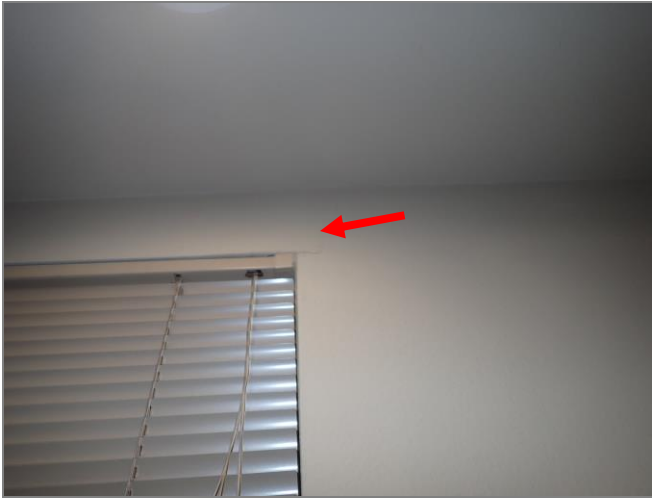
Additional cracking was observed in the interior drywall at the head of the window.
