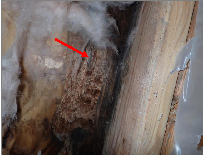
Water damaged exterior plywood sheathing was observed below the window sill corner.
