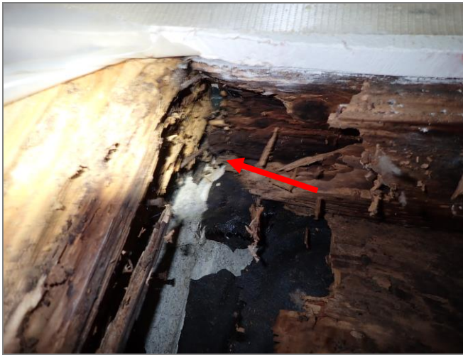
Water was observed entering at the window sill corner first (red arrow).
