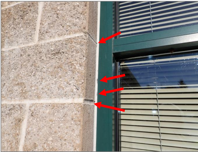
During the site visit performed on September 30, 2024, we observed some separation in the sealant joint at the west end window jamb (red arrows).
