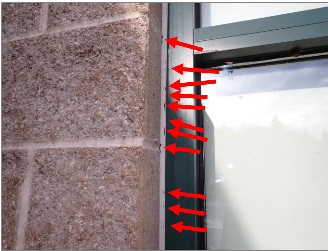
During the follow-up site visit, several openings were observed in the same sealant joint at the window jamb with the previously observed openings becoming larger (red arrows).
