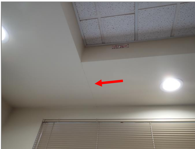
Stress crack in ceiling gypsum board was observed.
